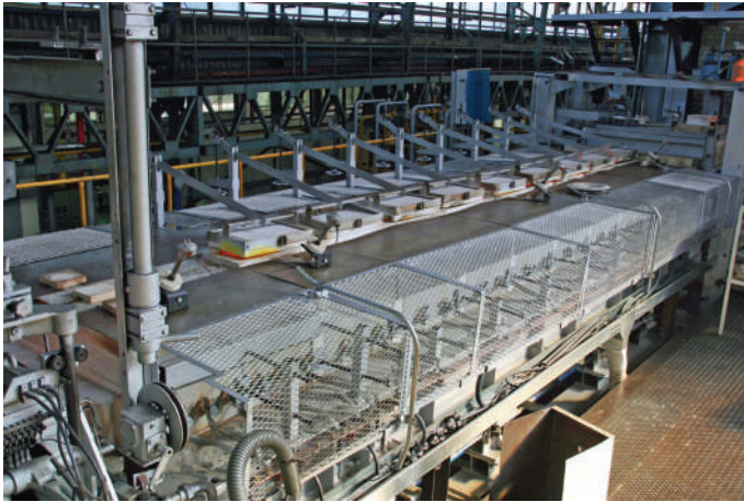
Figure 2-Typical Electroflex all-electric forehearth
