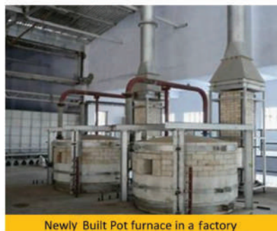
Newly Built Pot furnace in a factory
