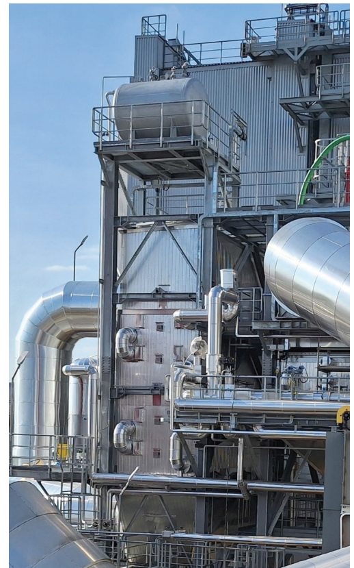
GEA supports its customers with extensive expertise and experience in waste heat recovery in the treatment of process gases. Numerous plants have already been equipped and retrofitted accordingly. (Photo: GEA)
