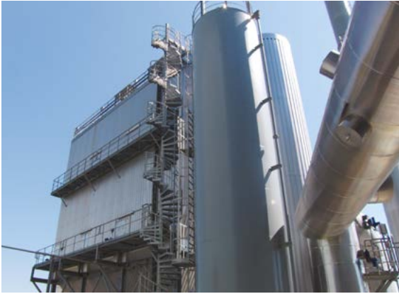
External view of the ZIPPE fully automated batch plant.
