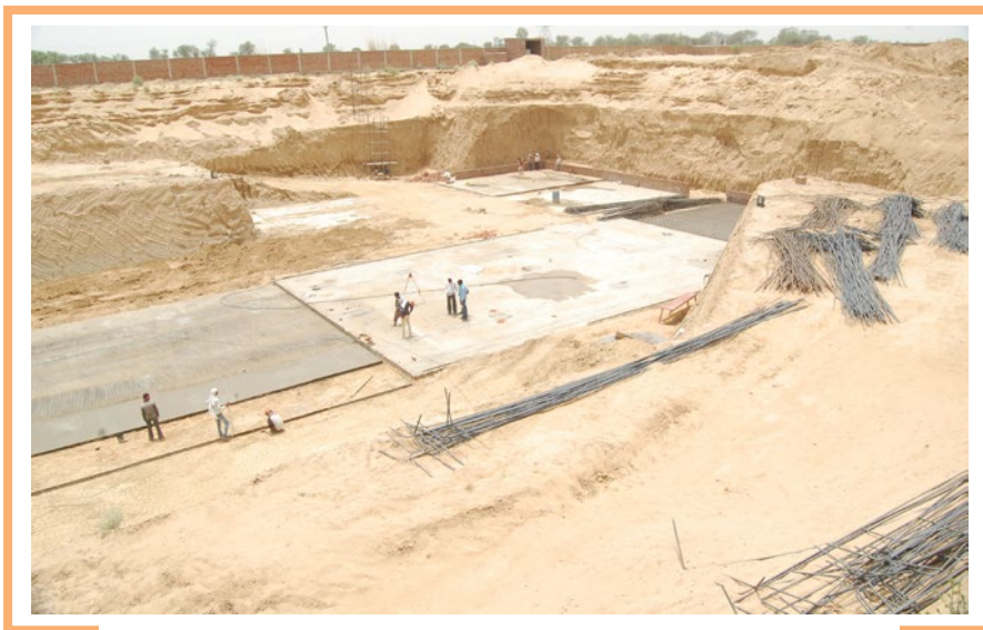
Ongoing Civil Work of EGIPL Plant at Keshwana Rajput Industrial Area, Tehsil Kotputli, Distt., Jaipur
