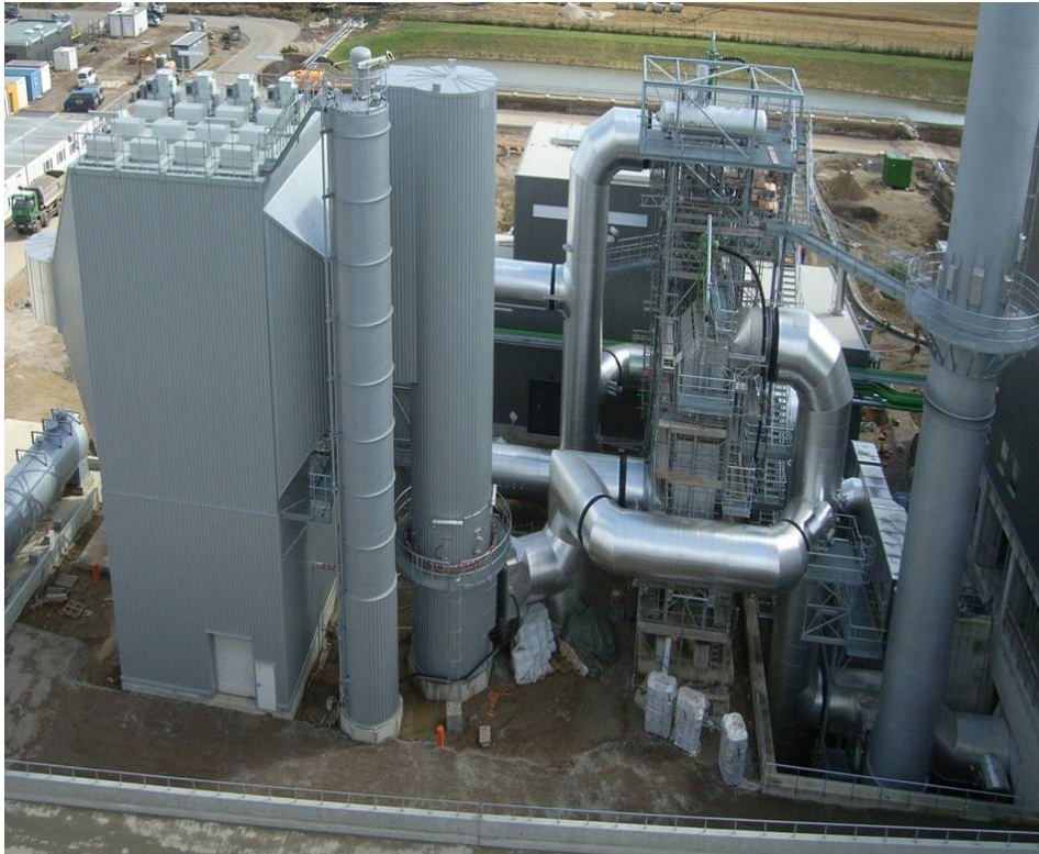
Combined WHR and Waste Gas Cleaning system
