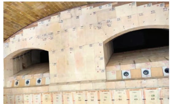
Furnotherm offers a comprehensive range of furnace construction services, including draining, demolition, rebuilds, heat-up, steelwork, refractory installation, utilities, electrical and instrumentation work.
