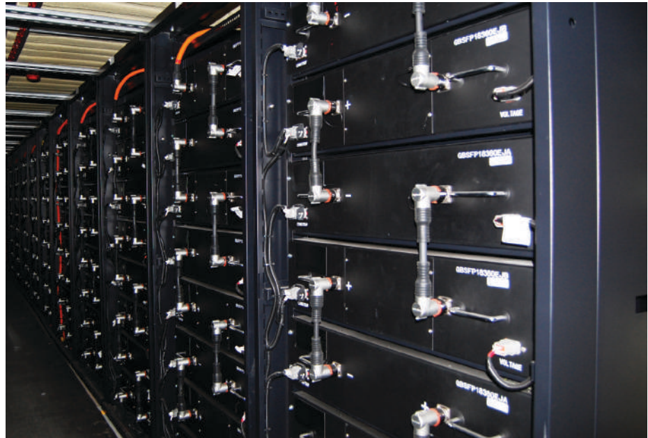
Inside a battery energy storage system (BESS).
