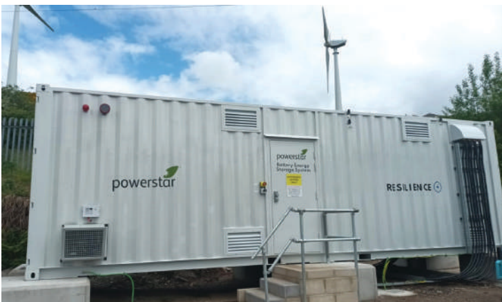
Parkinson-Spencer Refractories’ 250kW BESS provides an uninterrupted power supply in the event of Grid disruption.
