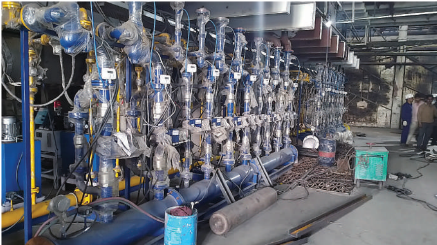
Along with the four container forming lines, Emerge has invested in forehearths from Shandong and Glass Era, who has also supplied furnaces.
