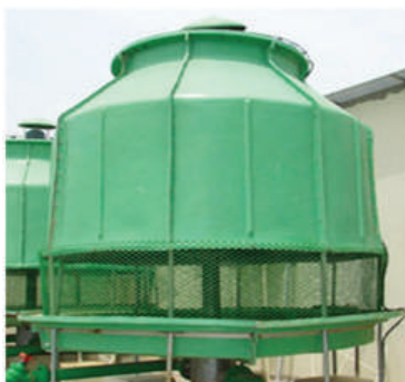
Fibreglass cooling towers
