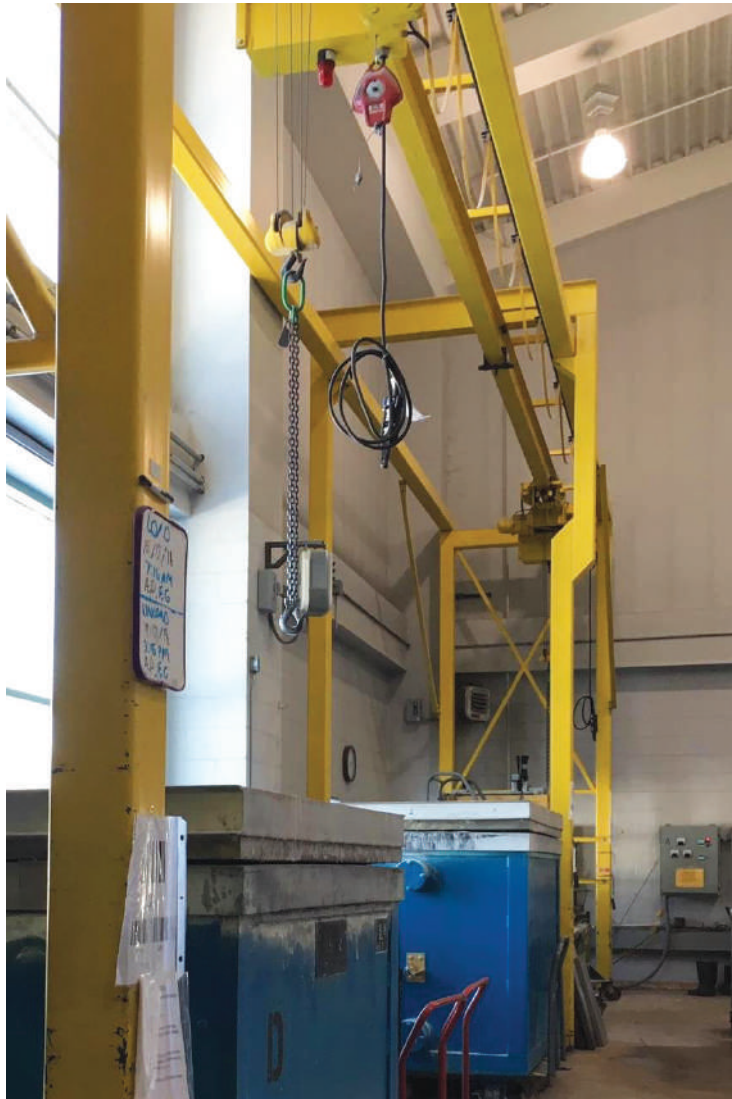
Crane set ups and molten salt tanks inside Saxon Glass Technologies.
